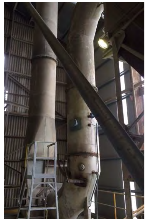
Figure 2: Cement Mill 2 Exhaust Duct
