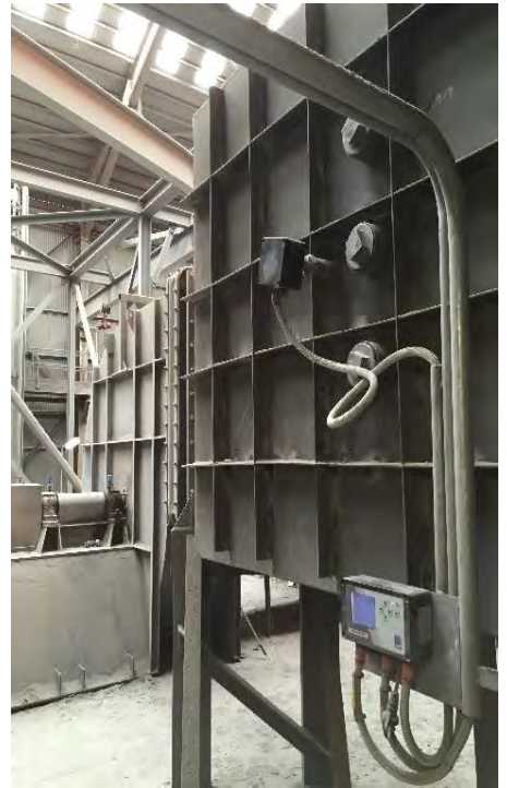
Figure 3: Cement Mill 3 Exhaust Duct
