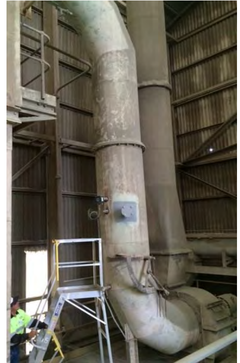
Figure 1: Cement Mill 1 Exhaust Duct
